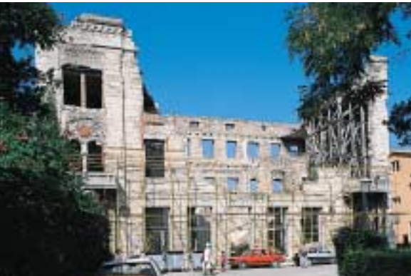
The photograph shows the street façade of the Vakuf Palace in its present condition. Most of the decorative elements were destroyed and will have to be reconstructed from the existing remains and the available documentation.
