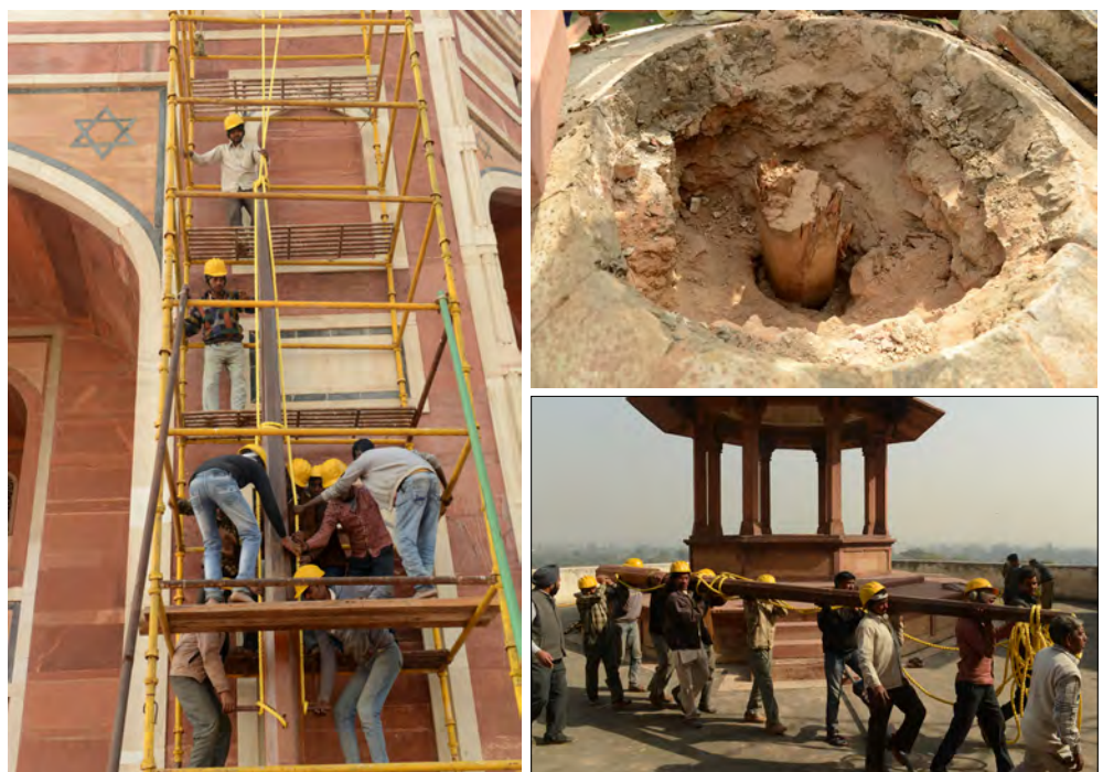
(Right) The 22 feet tall tree log being manually lifted to the dome of Humayun's Tomb. Since a significant portion of the wooden shaft was embedded in the dome masonry a tree log of 22 feet height was procured and carved to the original octagonal profile. In order to prevent repeated snapping, the base of the log was encased in a thin sheet of copper up till the top of the dome.
