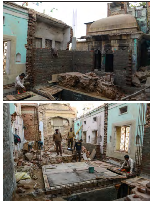
Work underway to reconstruct the Baoli arcade. This required the modern structure to be demolished and rebuilt 3 feet inside.
