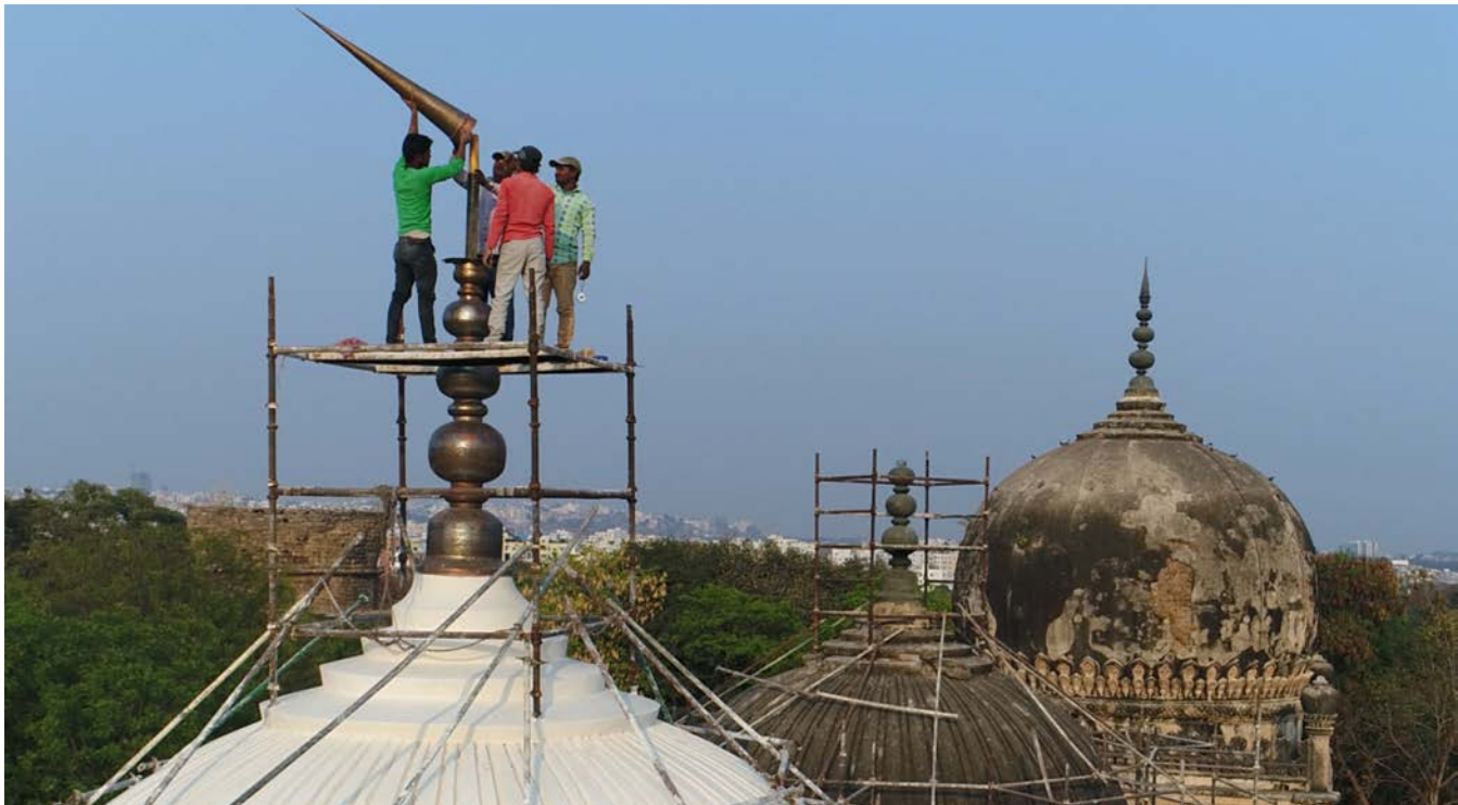
Installation of finial on the western dome of the twin mausoleums of Hakims'. (Top Left) Cement finial on the mausoleum to the west ; (Top Right) Local coppersmith fabricating components of copper finial; (Below) Installation of the finial on the dome
