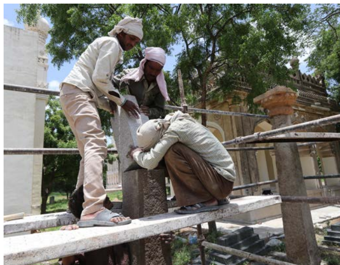
A hand carved stone piece of matching profile was retrofitted with stainless steel dowels along with epoxy resin
