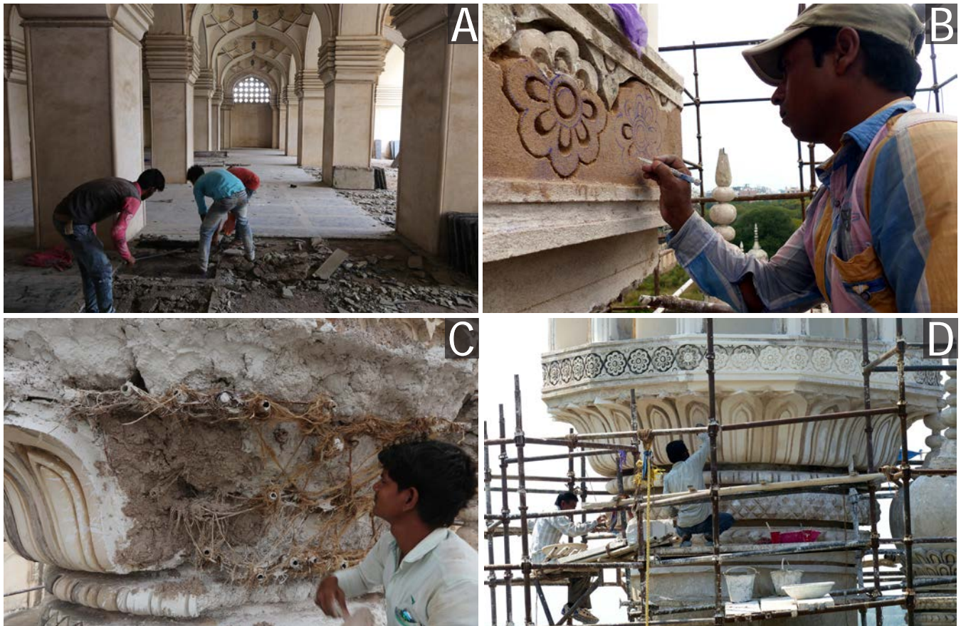
A: Dismantling of inappropriate 20 th century stone flooring; B: Carving of floral medallions by lime craftsman ; C: Reinforcing damaged portion of minarets with jute fiber and lime mortar; D: Finishing of restored floral brackets supporting the arch gallery
