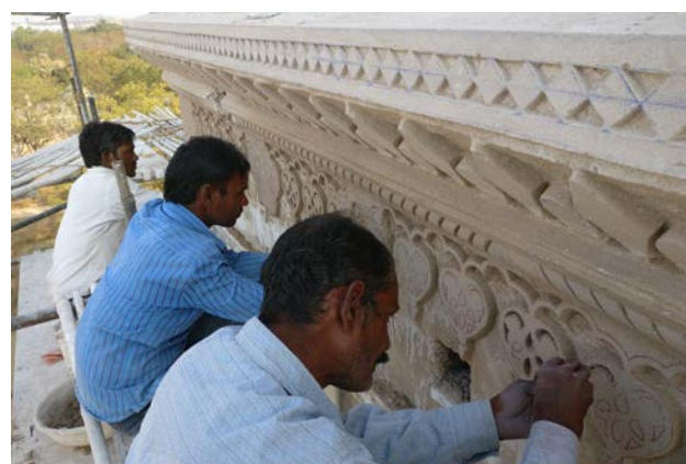
Conservation works were preceded by removing cement layers to reveal hidden tiles and stucco work - all of which have been well documented and consolidated to prevent ingress of water
