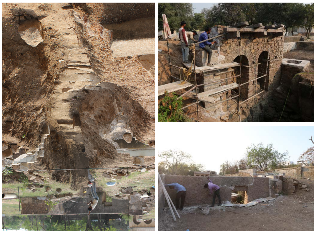
(Left) Aqueduct to the east of baoli; (Top right) Missing hand dressed edging stones on the western and southern ledge of the baoli were installed; (Bottom right) Low height brick parapet installed to prevent visitors from tripping inside the baoli
