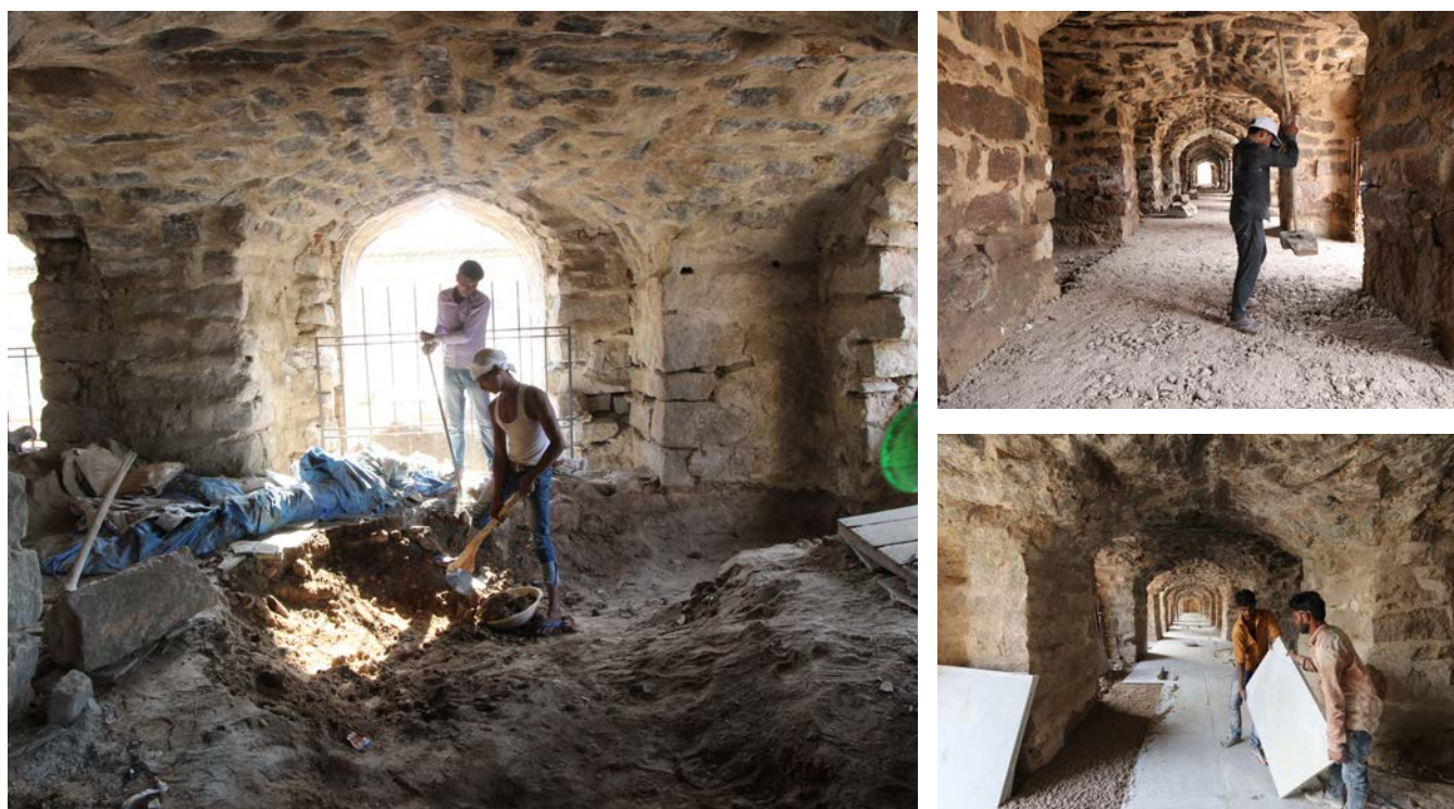
(Left) Removal of excess earth and debris; (Top Right) Lime concreting for installation of flooring; (Bottom Right) 30 mm thick granite stones laid
