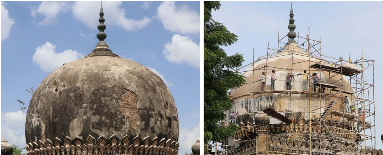
(Left) The dome of the mausoleum of Commander was covered with 20 th century cement plaster which was causing damage; (Right) After careful removal of the cement layers, lime plaster was applied on the dome.
