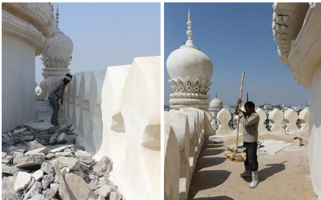
Removal of 20 th century cement layers from the roof of the mausoleum
