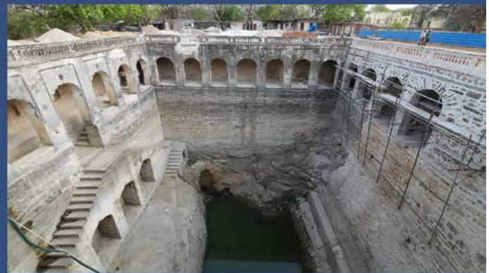
Existing stones from the collapsed western wall reused for repair of the wall.
