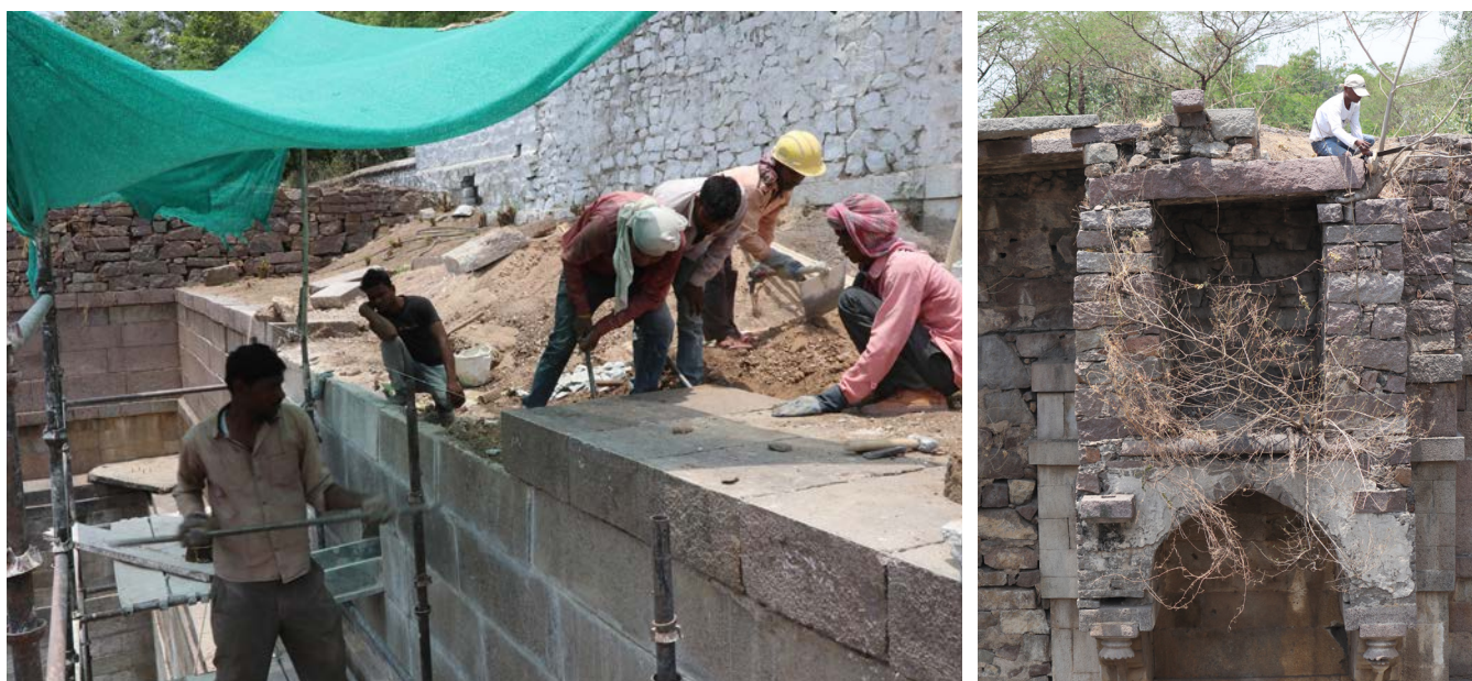
All the displaced dressed stones were realigned into place using the existing stones as reference Thick tree roots were removed carefully to mitigate any further displacement and movement to the stones.
