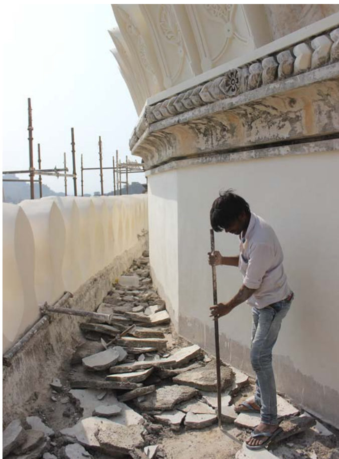
Removal of 20 th century cement concrete layers from the terrace of the mausoleum
