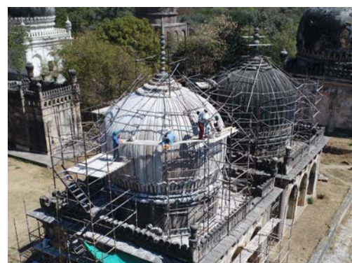
(Above) Restoration of the ribs on the dome of Hakims mausoleum in lime mortar
