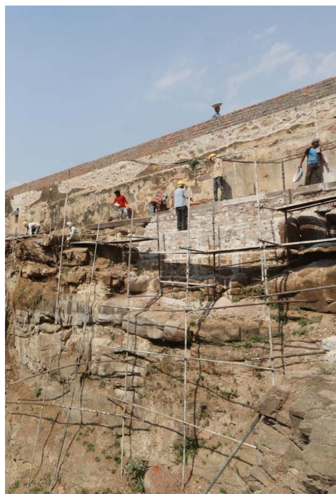
Missing hand dressed edging stones on the western and southern ledge of the baoli were installed
