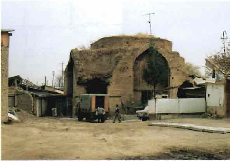
The Ak Sarai mausoleum remains the only monument in the area still engaged in the surrounding residential fabric. Until recently, the exterior niches of the structure were used by nearby houses as storage areas.
