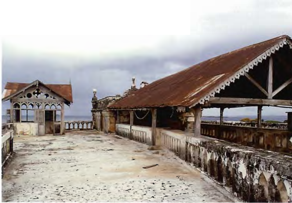
High roof level, with view of deteriorated stair bulkhead, courtyard, and roofs, prior to restoration.
