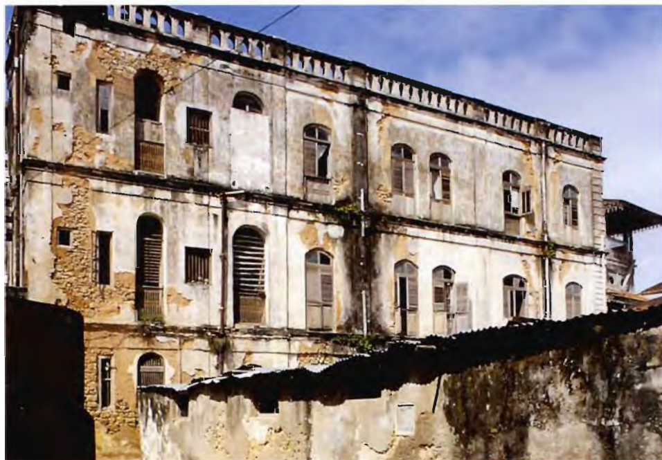
View of the north façade in 1990, indicating large areas of failed plaster work.
