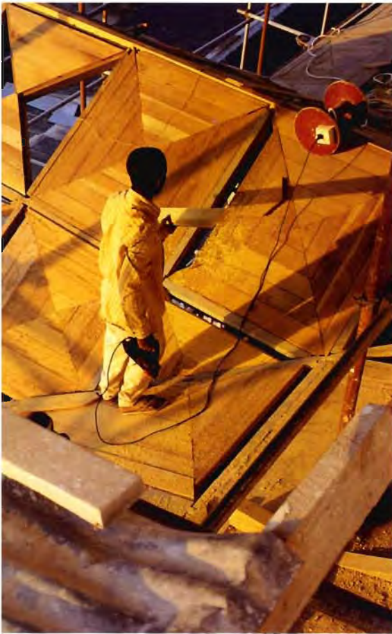
The roof of the second floor balcony under repair: The roof was reconstructed in its entirety, one half at a time.
