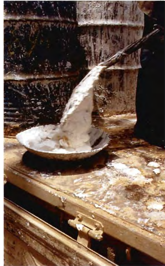
Lime production on site. The quicklime is slaked into cauldrons and then stored in tanks as putty until it is ready to be used.
