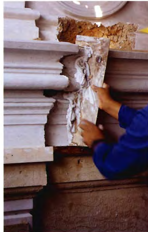
A fine coat of smooth, white finish plaster applied to a moulding.
