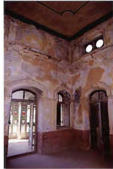
Interior detail of extensive plaster damage in the large cubical room, on the second floor.
