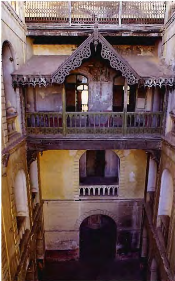
Interior view of the courtyard before restoration, showing severe deterioration of the base coat plaster walls, and timber balconies.
