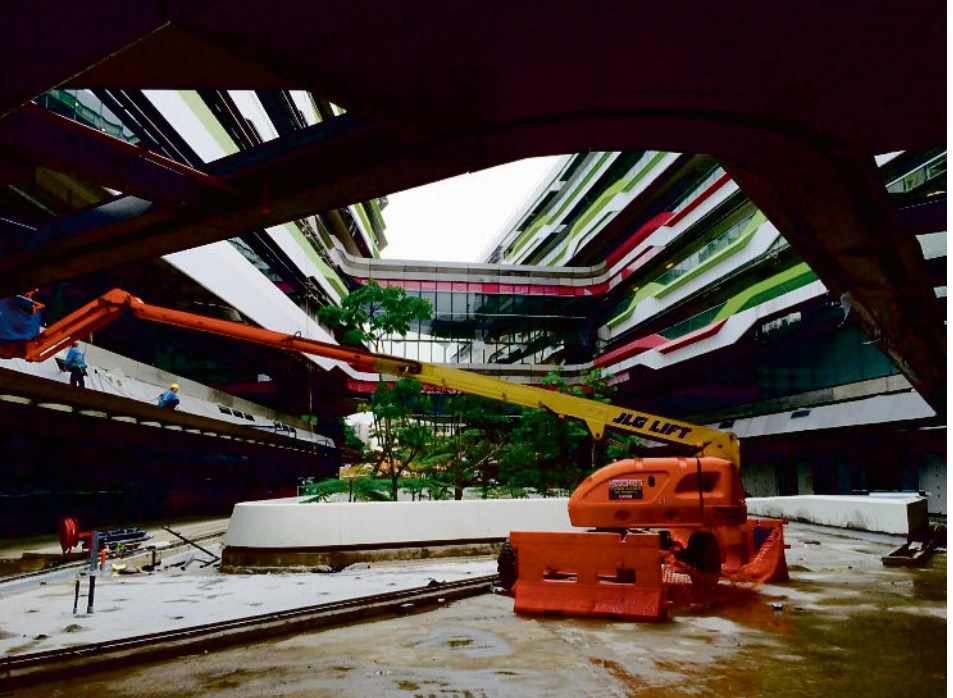
FIG. 4: SUTD, construction work taking place in November 2014. The master plan will be implemented through a series of architectural design competitions. The academic core complex, shown under construction in this image, was designed by UN Studio of the Netherlands and was completed in 2015
