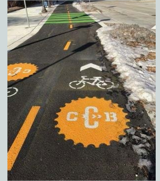
Figure 92: Image showing Permeable Pavements along Jackson street, St. Paul
