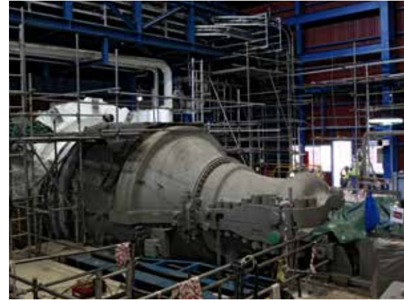
Above and below: The Azito Energie power plant generates 25-30 percent of Côte d'Ivoire's electricity production.
