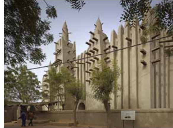
Above and below: Following the signing of the Agreement of Cooperation between the Government of Mali and the AKDN in 2003, the Aga Khan Trust for Culture began its Earthen Architecture Programme by restoring the Great Mosque of Mopti, also known as the Mosque of Komoguel. These photos show the Mosque after restoration.
