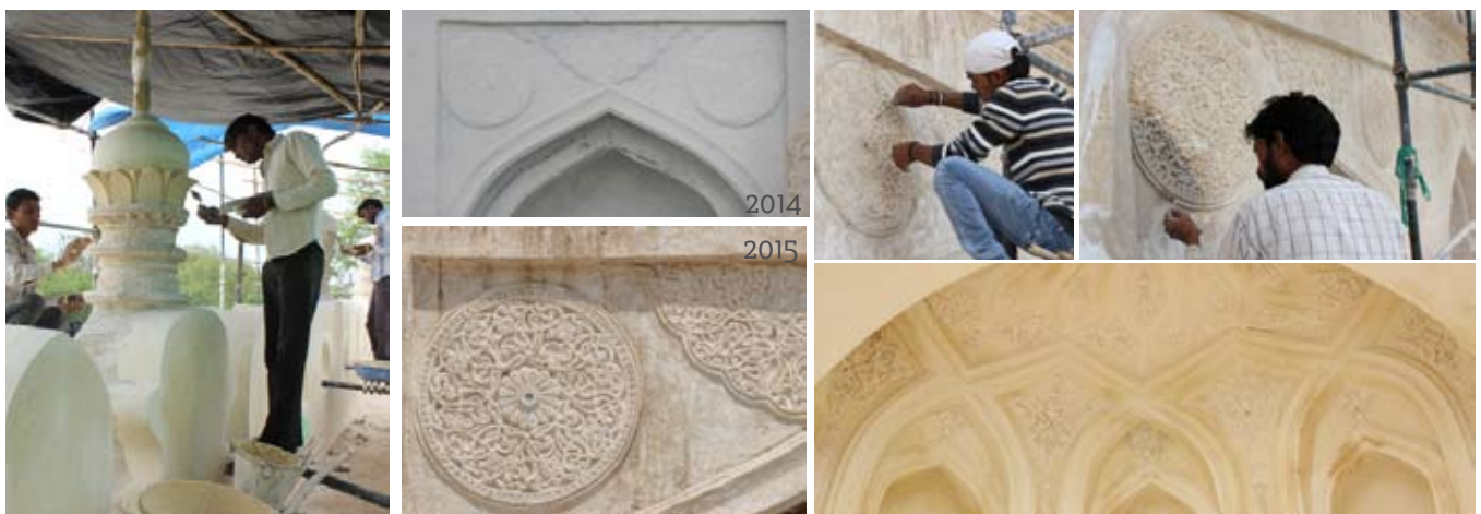
Restoration of ornamental incised lime plasterwork after removal of 20 th century paint layers
