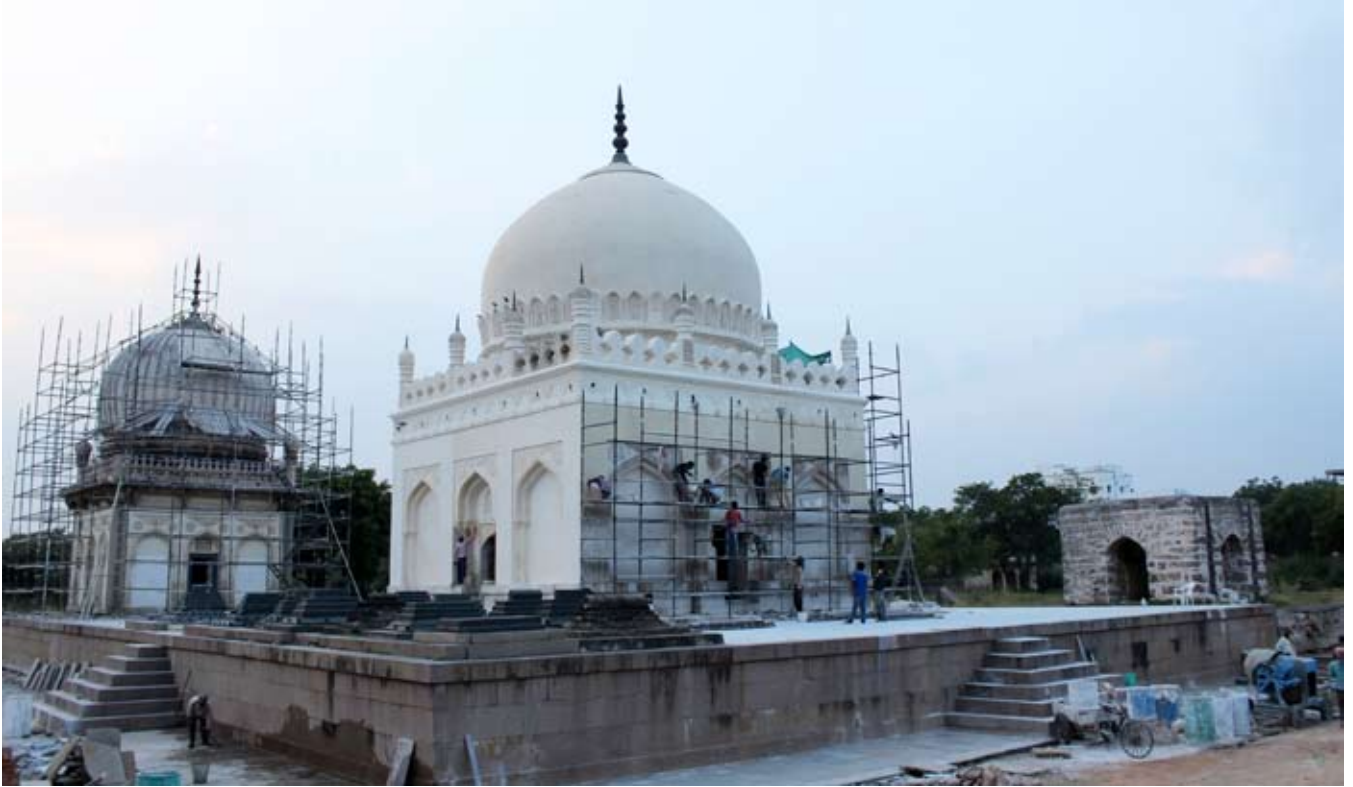
(Above) Conservation works on Sultan Quli Qutb Shah's Tomb required replacing cement plaster with traditional lime plaster and conservation works now commencing on Subhan Quli Qutb Shah's tomb will aim to achieve similar results
